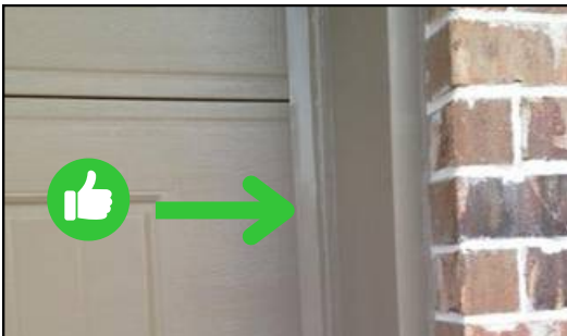
Garage Door Weather Stripping
