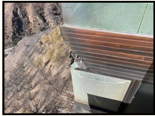
A scorched hillside leading up to a damaged deck. Credit: Cal Fire's Damage Inspection files from the 2025 Palisades Fire.
